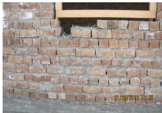
Photo 2 - School Building's Exterior Brick Wall with Gaps in Mortar
