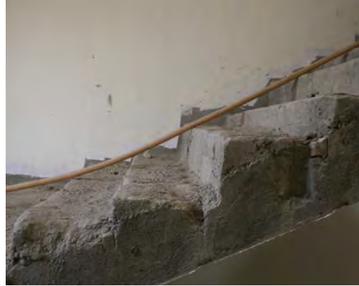
Photo 3 - Stairs of Different Heights and Crumbling at Garm Ser Site
