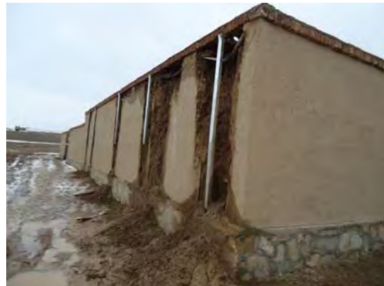
Photo 1 - Exterior View of Building Deterioration Due to Water Penetration
