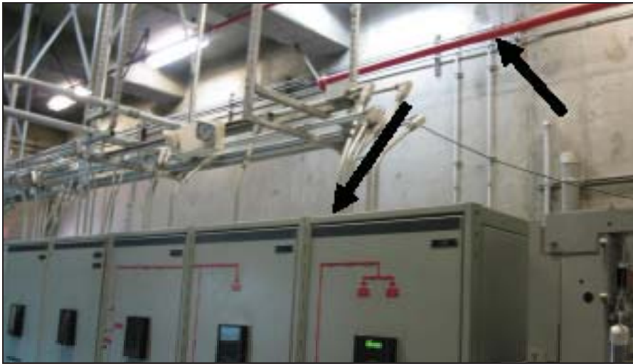
Figure 4: This photo shows the sprinkler system (up arrow) above the switchgear (down arrow) in the west compound.
