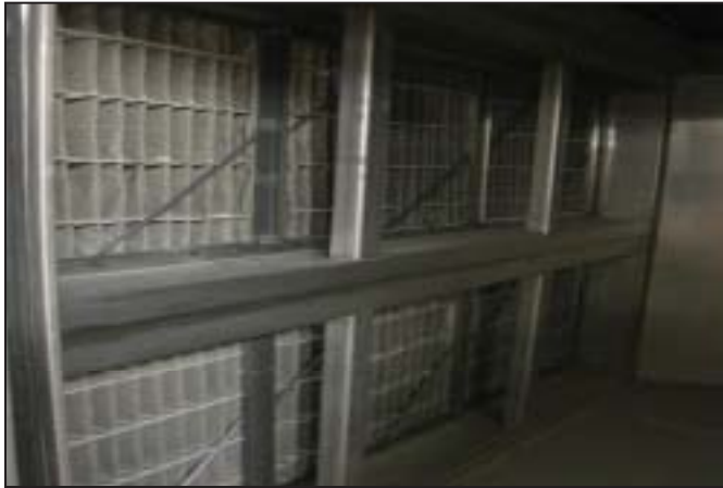
Figure 5: This photo shows pre-filters inside a heating and air conditioning unit.
