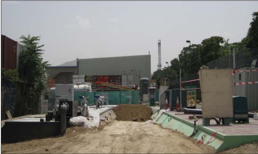
Figure 3: This photo shows sewage tanks on Embassy Kabul's west compound.
